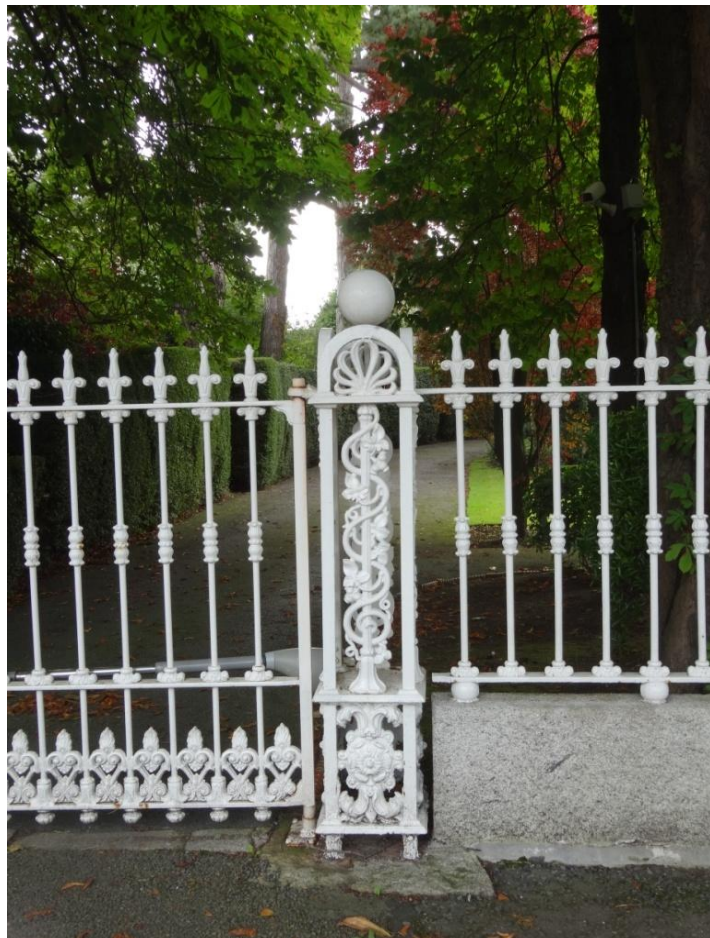
A decorative cast-iron gate post is set between the gate to the left and a granite plinth wall with railings to the right. The mid-19 th -century gates have been mechanised.
